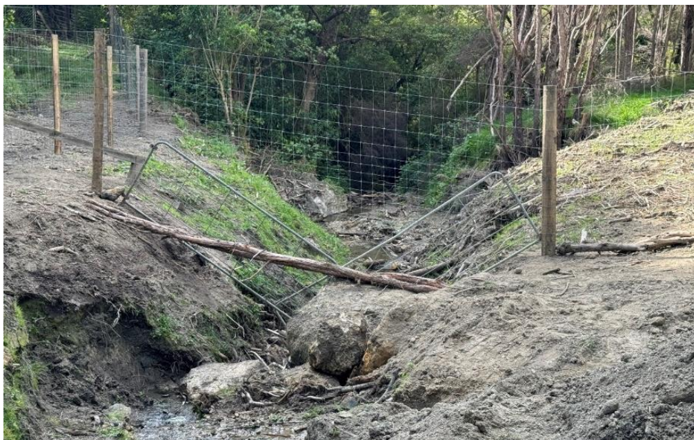
Figure 11: Repaired section of deer fence in the Pākuratahi HCV / QEII block. This was a significant blow out and required extensive woody debris removal.
