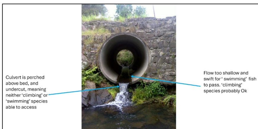
Figure 20: A typical perched culvert showing multiple aspects of barrier to migration. This culvert would be impassable to any fish species
